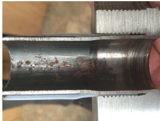
Corrosion of a carbon steel tube.
