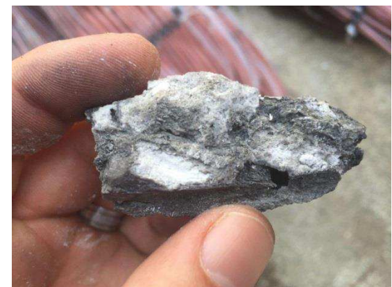
Fly Ash build-up retrieved from the tubes during maintenance.
