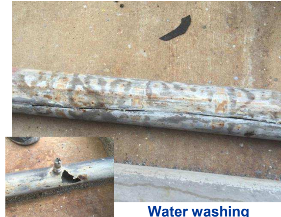
Wear damage of carbon steel tube.
